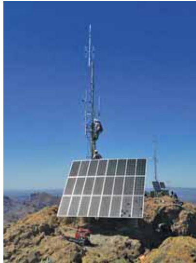
An LMR solar site shows the pre-staged P25 station installed at a typical remote site node.
